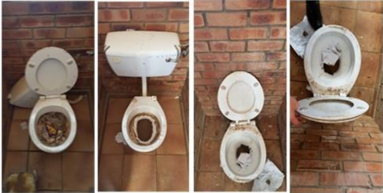
Figure 1. Conditions of the toilets for students at School A on the first site visit.
