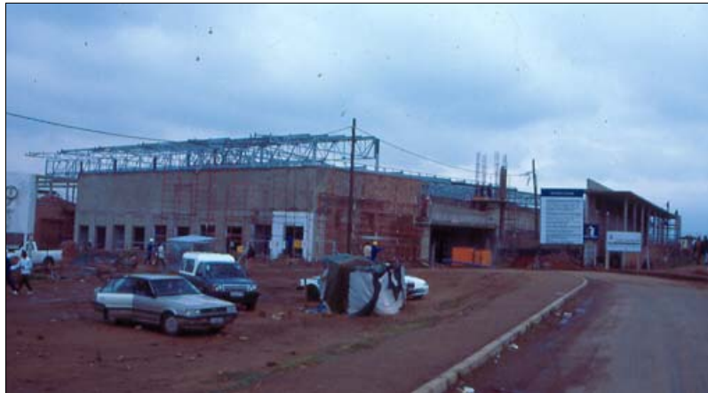
Illustration 3: Construction underway in Kliptown as part of developing the Walter Sisulu Square of Dedication, where the Freedom Charter was adopted in 1955. Photograph: S. Marschall, 2004.
